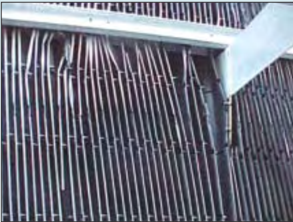
Other manufacturers' – Gaps in Eliminators on Hanging Fill Sheets
