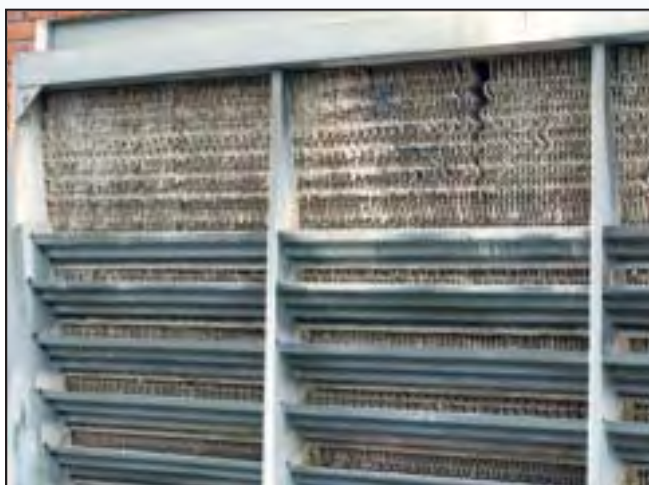
Old, Inefficient, Damaged Fill
